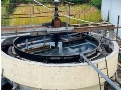
Effluent Treatment Plant
